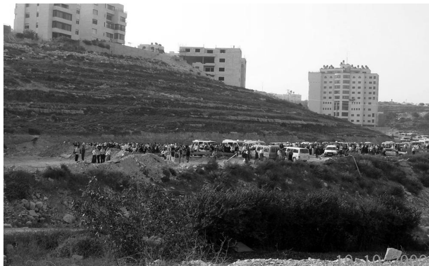
Photo 4: Birzeit – Ramallah road trenched and closed with embankment at two locations about one kilometer apart, forcing all passengers to depart transit vehicles and walk for about one kilometer and ride vehicles on the other side of the road closure, October 2002
